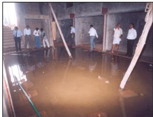
Stagnant water at construction site
