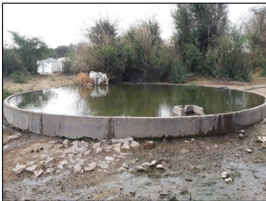
Surface water tank
